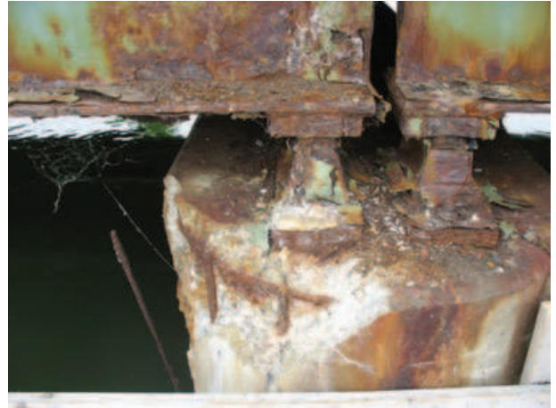
Fig. 13. Corroded bearings at the northern-most pier of the bridge.
