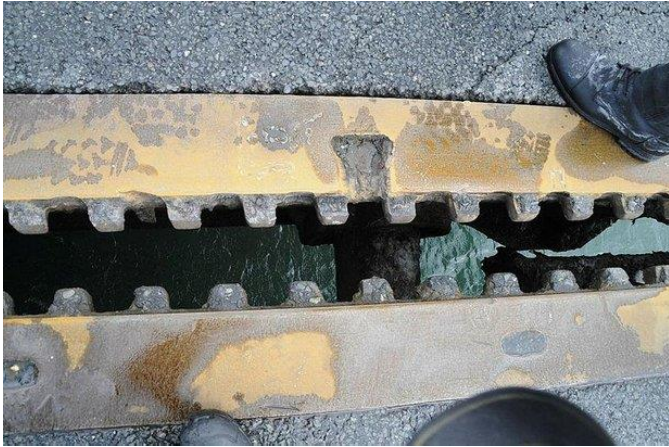
Figure 2. A closeup view of gap at the connection in deck.
