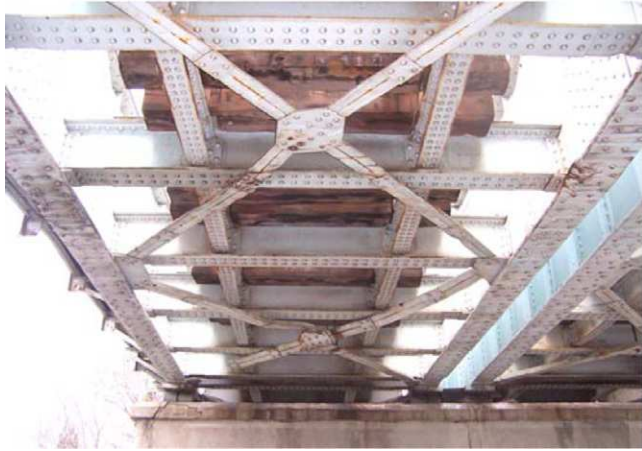
Fig. 3. Buckled cross braces under the fourth span.
