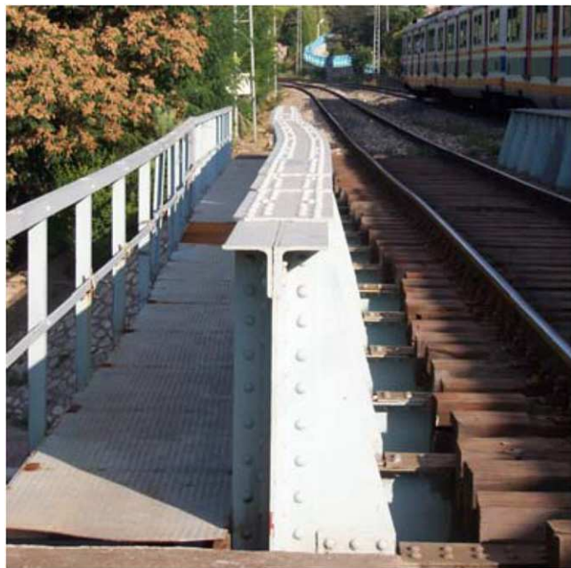
Fig. 4. Deformed main girder of the fourth span.
