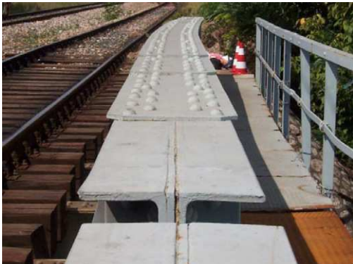
Fig. 29. Deformed main girder of the fourth span.
