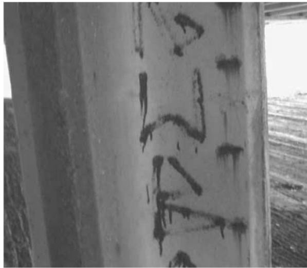
Figure 8: Insufficient concrete cover and stirrups corrosion
