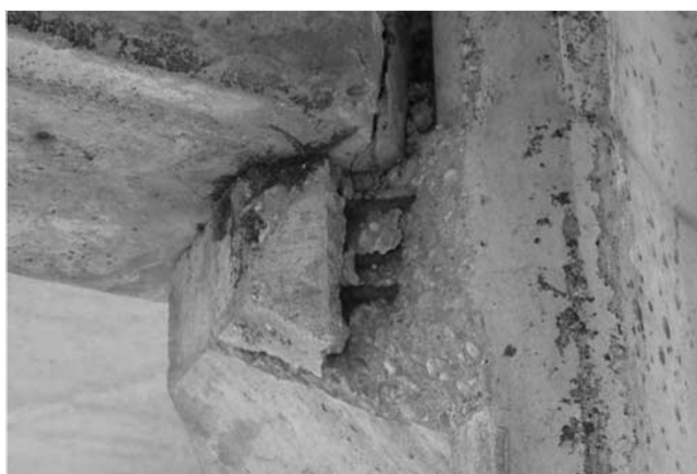
Figures 15: Separation of cover from column corbels (thick cover and poor reinforcement arrangement)
