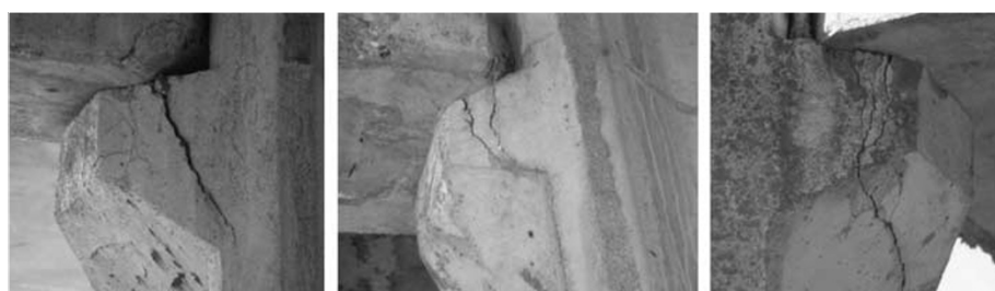
Figure 17: Oblique and vertical cracks
