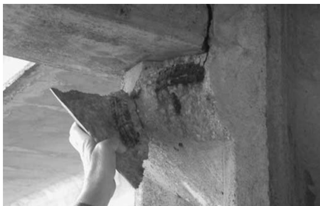
Figures 16: Separation of cover from column corbels (thick cover and poor reinforcement arrangement)
