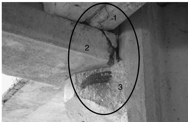
Figures 22: Oblique cracks in the resting places of ribs of the \Pi slab
