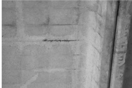
Figure 20: Defects and damage of \Pi slabs
