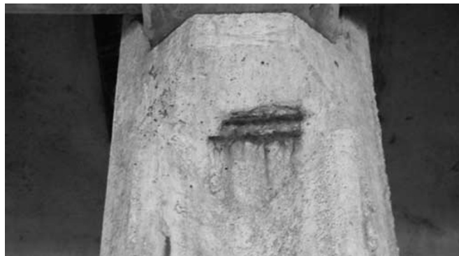
Figures 14: Insufficient concrete cover on column corbels
