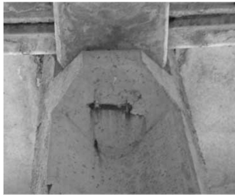
Figures 13: Insufficient concrete cover on column corbels
