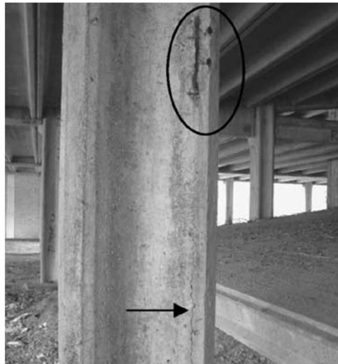
Figure 9: Corrosion of main reinforcement and longitudinal crack in column
