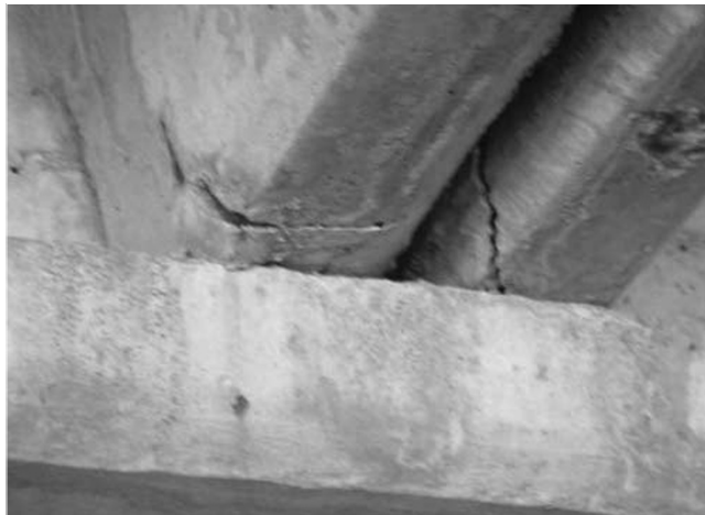
Figures 21: Vertical cracks in the resting places of ribs of the \Pi slab
