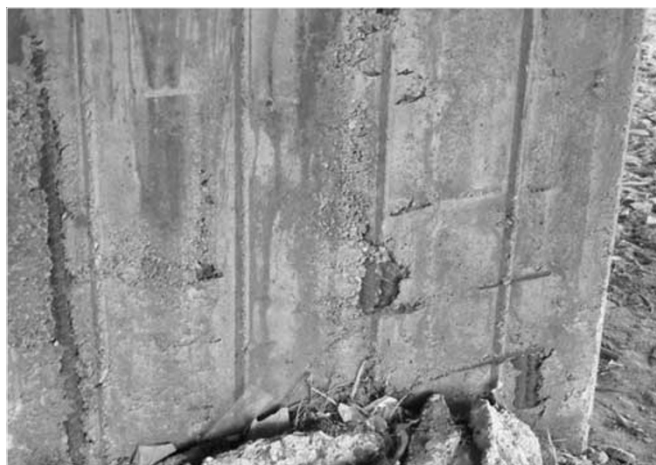
Figure 23: Defects in RC wall
